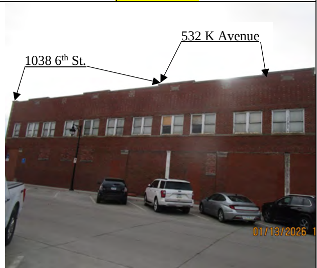
Alternate view of exterior of 1038 6 th St. and 532 K Ave. Windows and vertical columns with white paint tested positive for LBP.
