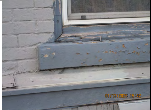
View of 2 nd level windowsill which tested positive for LBP .
