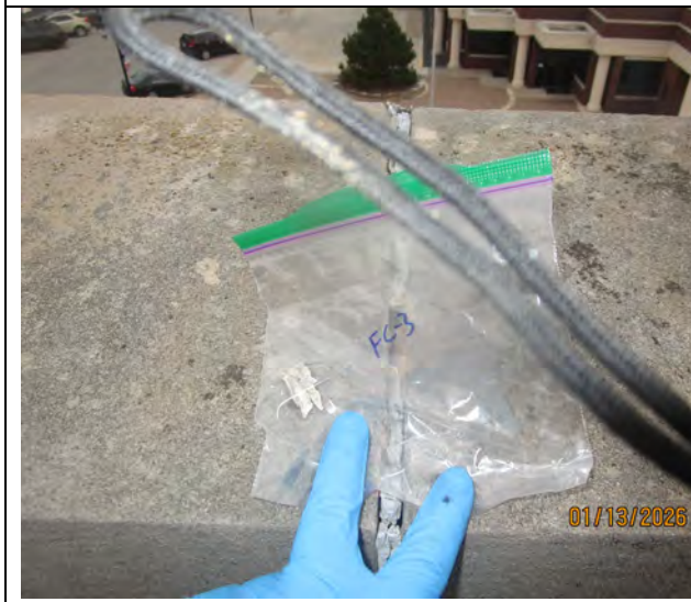
View of sample FC-3: Caulk between coping stones on parapet wall. 3% chrysotile asbestos.
