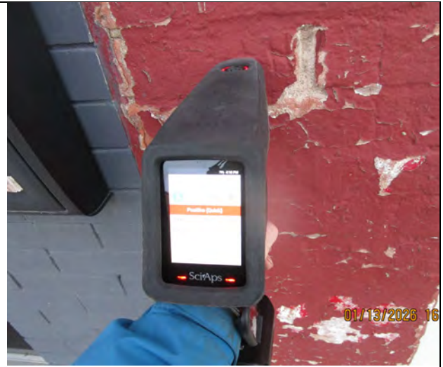
View of painted brick on lower level testing positive for LBP.
