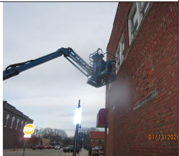
View of window caulking/glazing sampling: Window glazing samples WG-1 and WG-2 did not contain asbestos. Window caulk samples WC-1 and WC-3 tested positive for 3% chrysotile asbestos.
