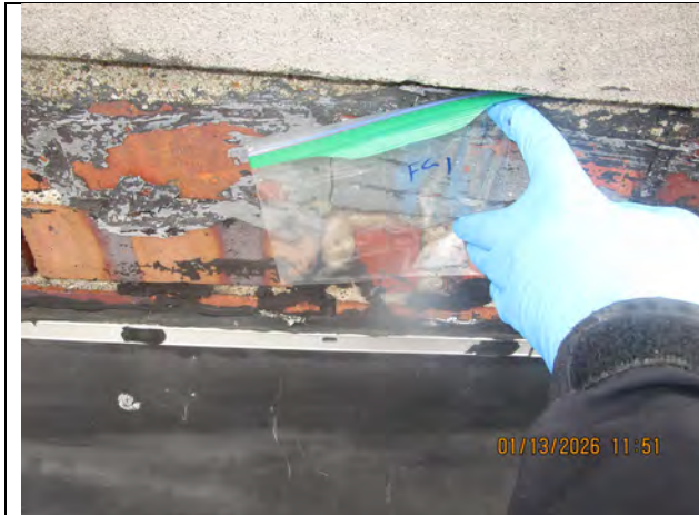
View of sample FC-1: Grey flashing cement on parapet wall. 8% chrysotile asbestos.
