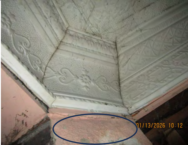
Corner column under pink paint, shown here above suspended ceiling tile, tested positive for LBP. White plaster and metal decor not positive.
