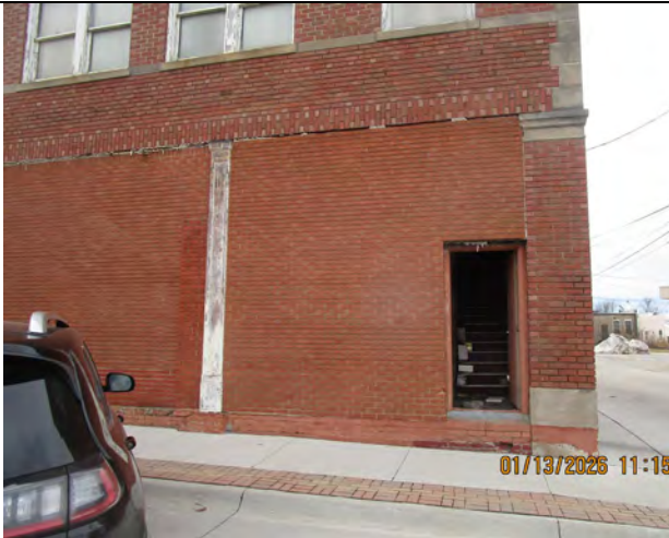
Structural column shown tested positive for LBP . Windows above also tested positive for LBP
