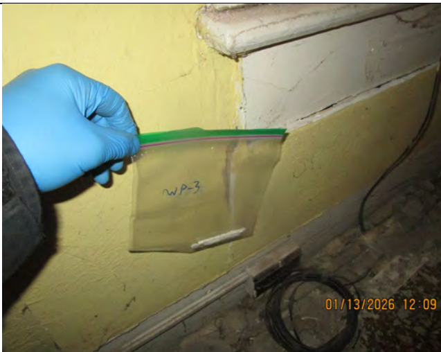
View of sample WP-3: Wall plaster with skim coat/texture on second floor. 2% chrysotile asbestos.
