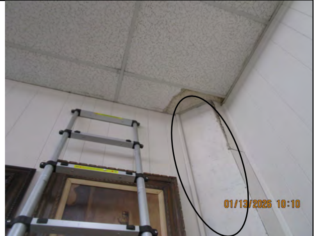
NE corner shown (street level); drywall & wood partially covering concrete column which is positive for LBP.
