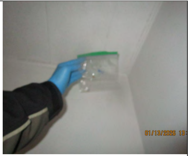
View of sample DW-1: Textured drywall ceiling in unit #2. 2% Chrysotile asbestos.
