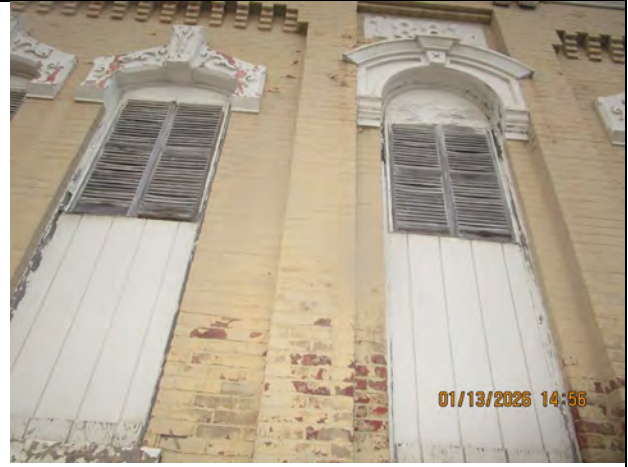
View of 2 nd level window components and architectural arches which tested positive for LBP.
