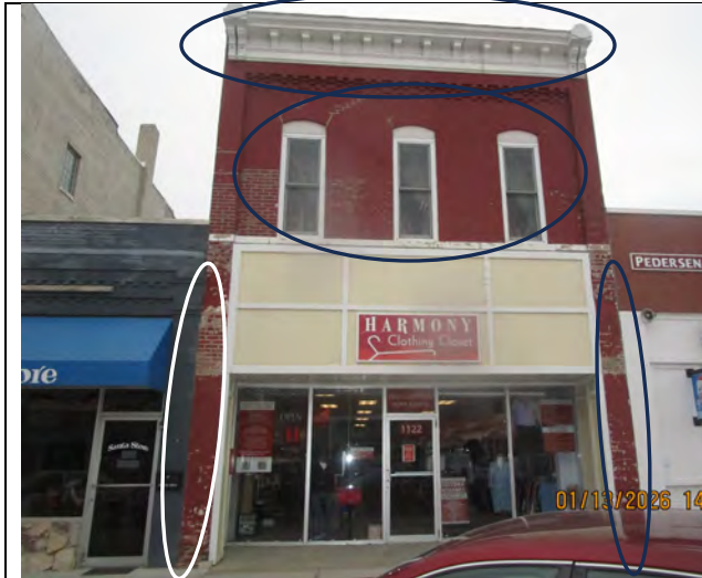
View of subject property, looking west. Both levels occupied by Harmony Clothing. Upper level windowsill / soffit and arches positive for LBP.
