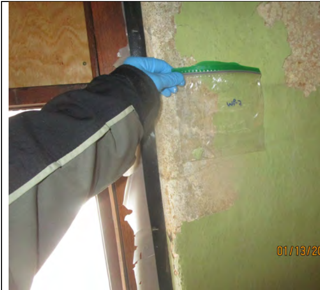
View of sample WP-2: Wall plaster with skim coat/texture on second floor. 2% chrysotile asbestos.
