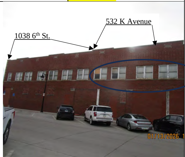
Alternate view of exterior of 532 K Ave. Windows and vertical columns with white paint tested positive for LBP .
