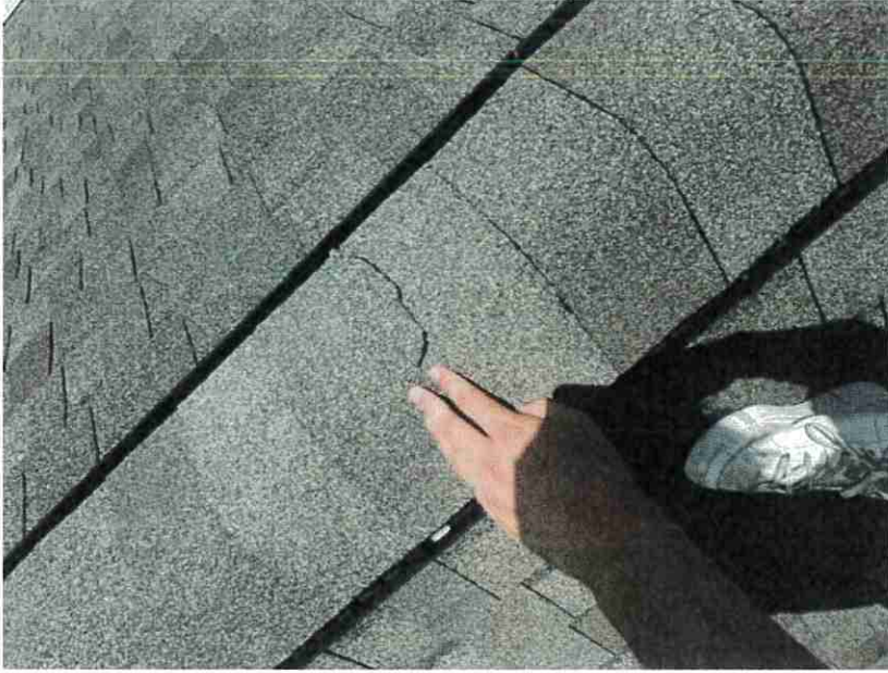
Ridge Damage (Included in both of our quotes below)
