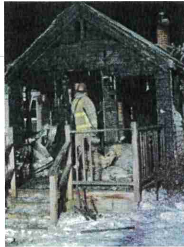
Fire-damaged house prior to demolition
